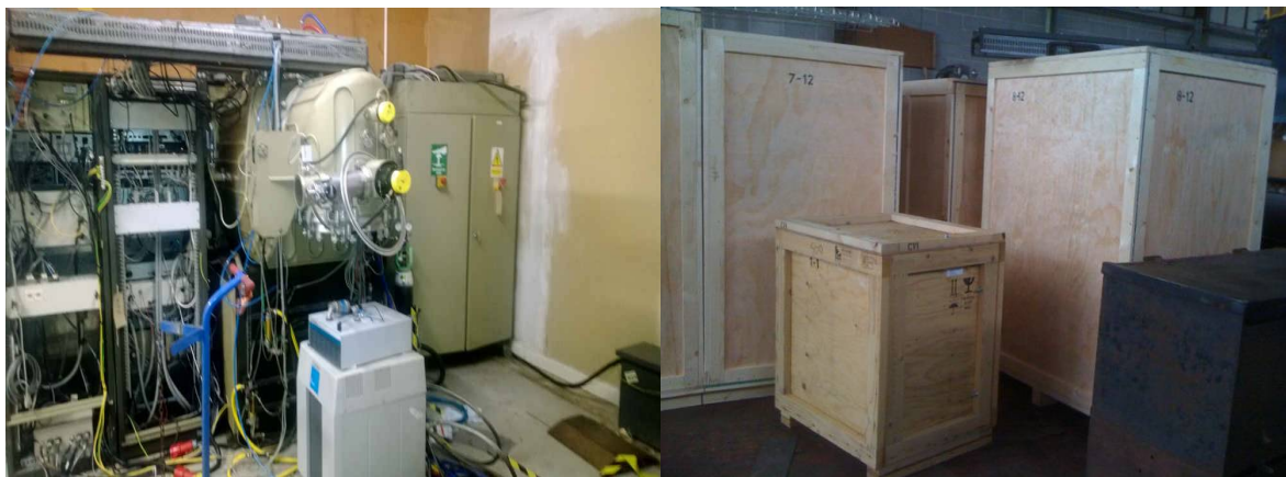
A typical 40 year old BAK760 coating system
